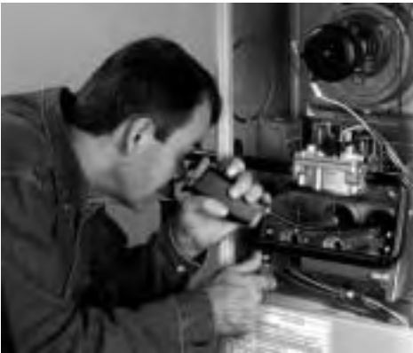
Fig. 22: Maintenance and inspection of heating unit without need for dismantling when testo 318 is used
