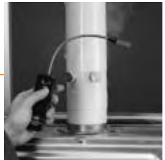
Flue gas spillage test using testo 317
