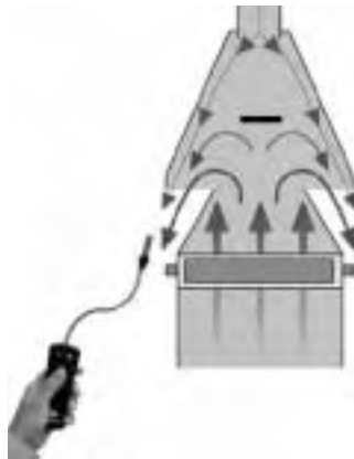
Fig. 21: Detection of escaping flue gases in the flow control unit using the testo 317-1 spillage detector
