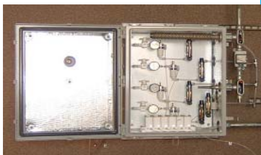
Sampling system for wet chlorine (above) has teflon valves and multipoint. sampling system is heated to prevent condensation. The sampling system valves are controlled by air actuated valves in the 301C.
